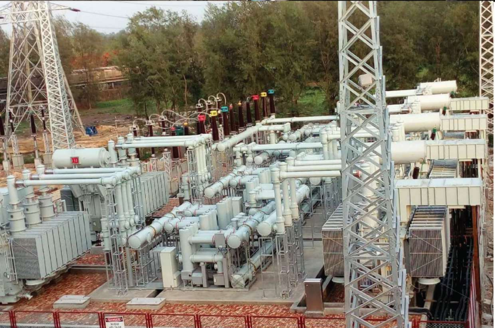
Sub Station Project 300 feet, Purbachal
